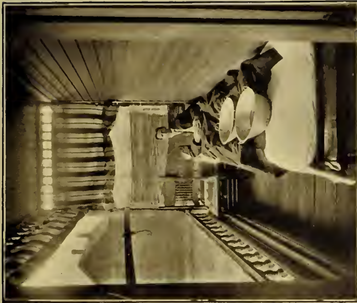
SEEKING FRESH AIR UNDER DIFFICULTIES—THE PANS ARE SET TO CATCH WATER FROM A LEAKY ROOF
